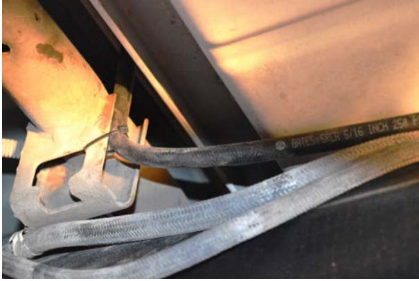
(Fig. 7) One of the vent hoses routed up and attached to the vehicle's body with quick tie.
