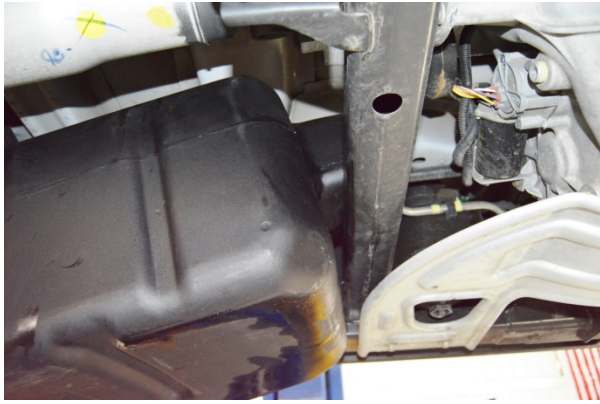
(Fig. 11) Angle tank slightly as it is lifted in so that front protrusion on tank slides over cross-member.
