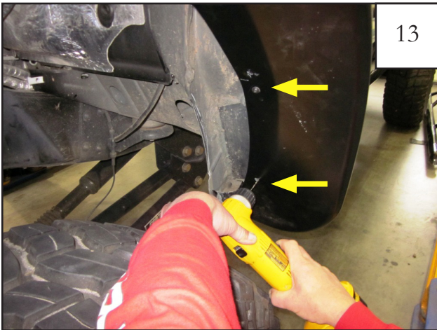
Hold flare tightly against fender, lining it up along style lines, drill into sheet metal through pre-drilled flare holes at rear side using 1/8" drill bit.
